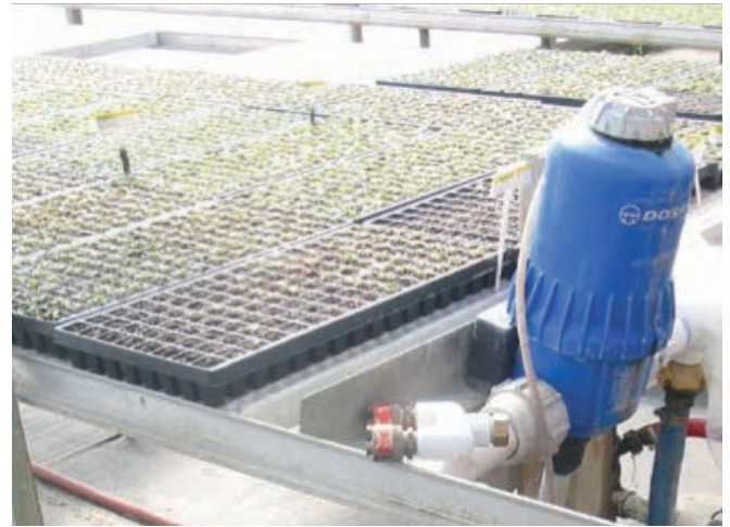
Dosatron injecting treatment solution into an irrigation boom.
